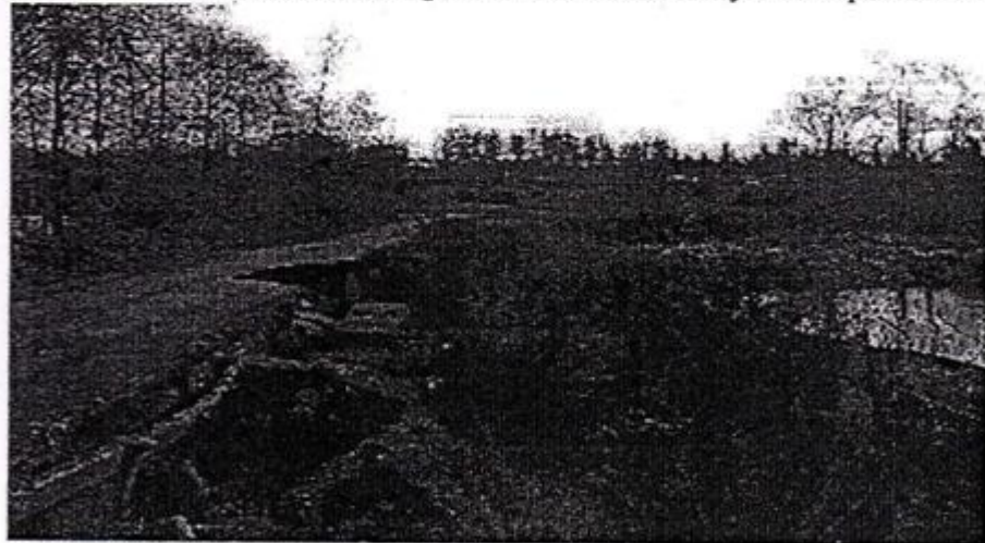
Figure 3 Flow failures in highway fill, Lake Merced, 1957 Daly City earthquake.
